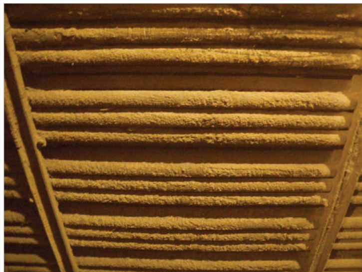
Figure 5. Fouled pre-heater coils.
